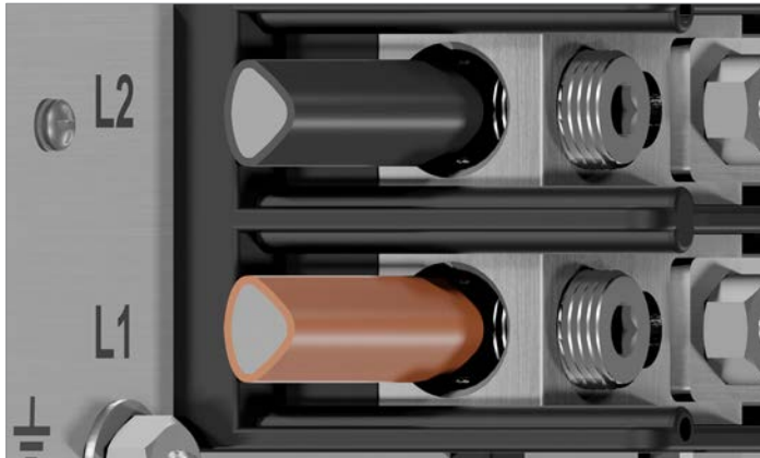
Fig. 7.12: Correct position of sector-shaped aluminum cables (2)
