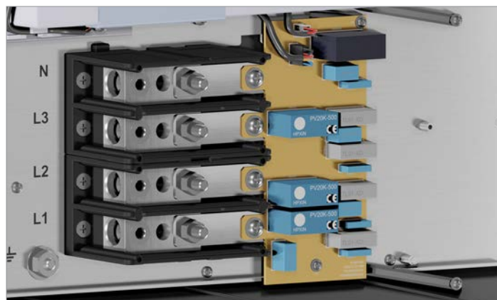
Fig. 4.5: View of type 2 AC surge protection devices with the cover removed
